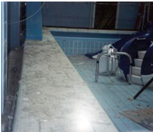
Figure 1.7 Uncontrolled removal of asbestos
