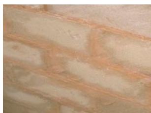
Figure 7.26 Remnants of asbestos on breeze blocks
