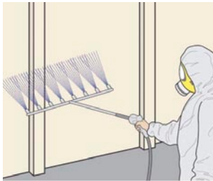
Figure 7.14 Multi-point spray system
